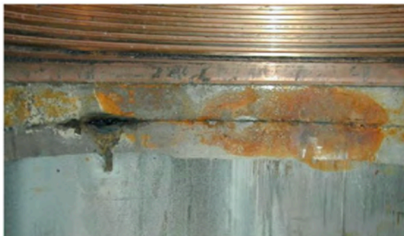
Fig. 5.6: Oil and gas pipeline under crevice corrosion
