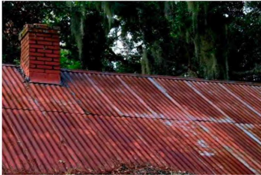
Fig. 5.4: UNIFORM CORROSION OF METAL ROOF
